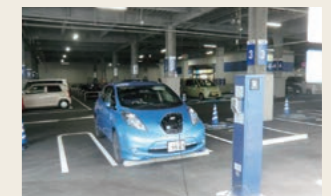
Charging spots for electric vehicles
